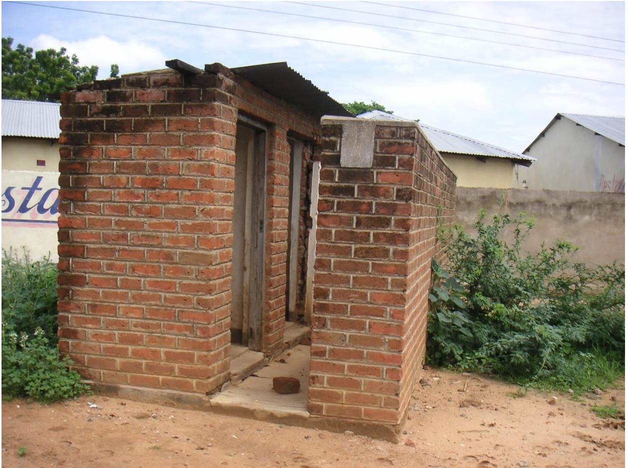
One of the toilets at New Bangula Market (not yet handed over to market users)
